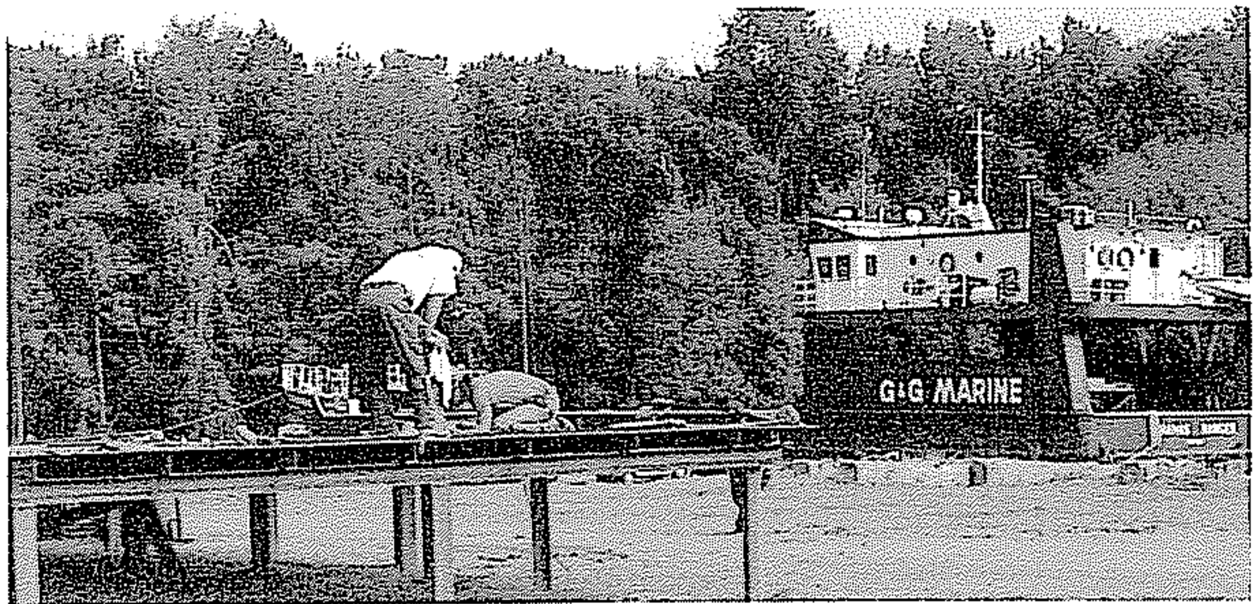
Steel workers build the first deck of the 160 foot offshore service vessel under construction at St. John's Shipbuilding.
